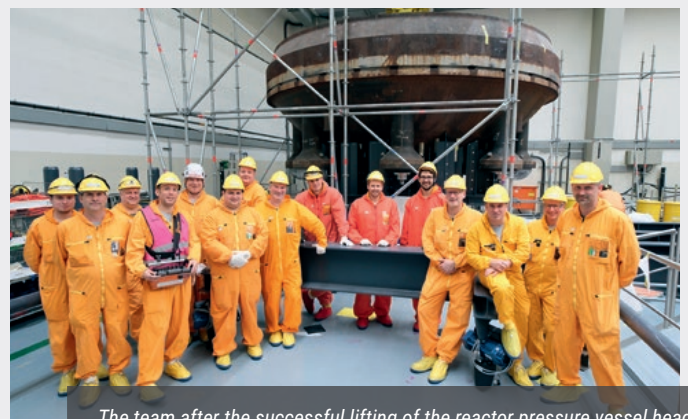
The team after the successful lifting of the reactor pressure vessel head.
