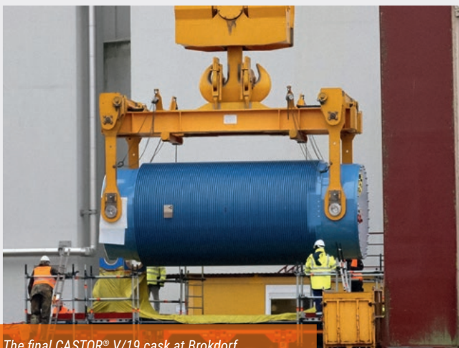
The final CASTOR® V/19 cask at Brokdorf. Photo: PreussenElektra GmbH.
